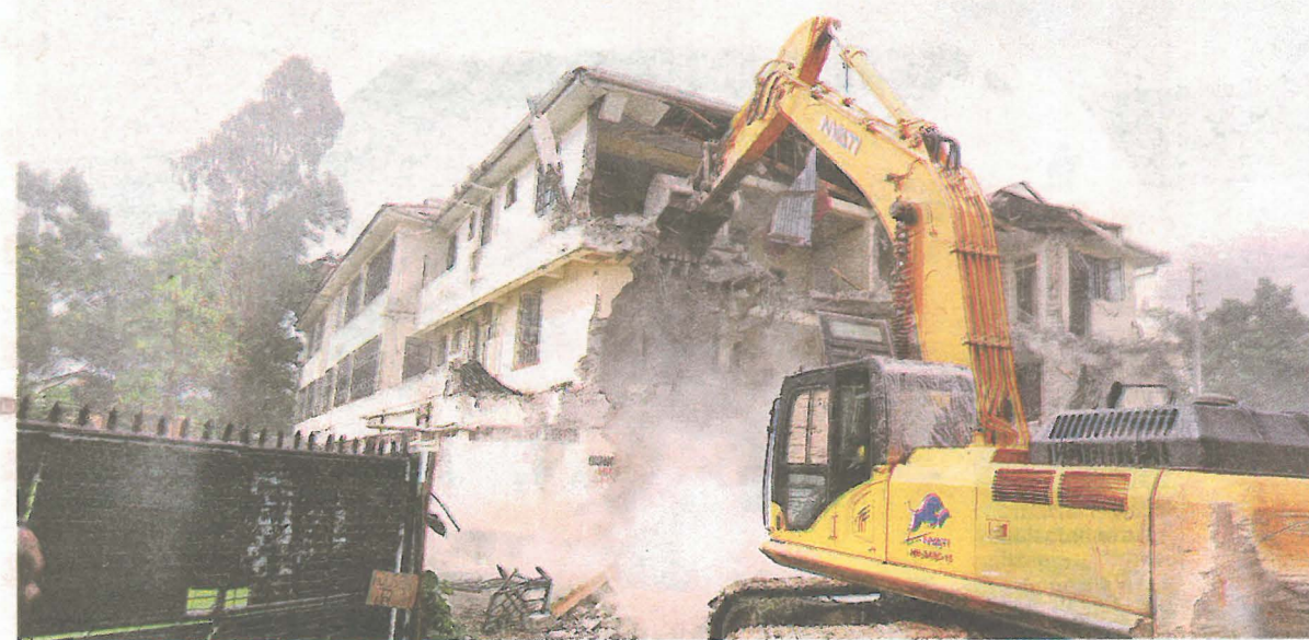
A bulldozer razes down a rental house in Migosi estate, Kisumu County in 2021. The house is said to have been constructed on the city's sewer line. [File, Standard]
